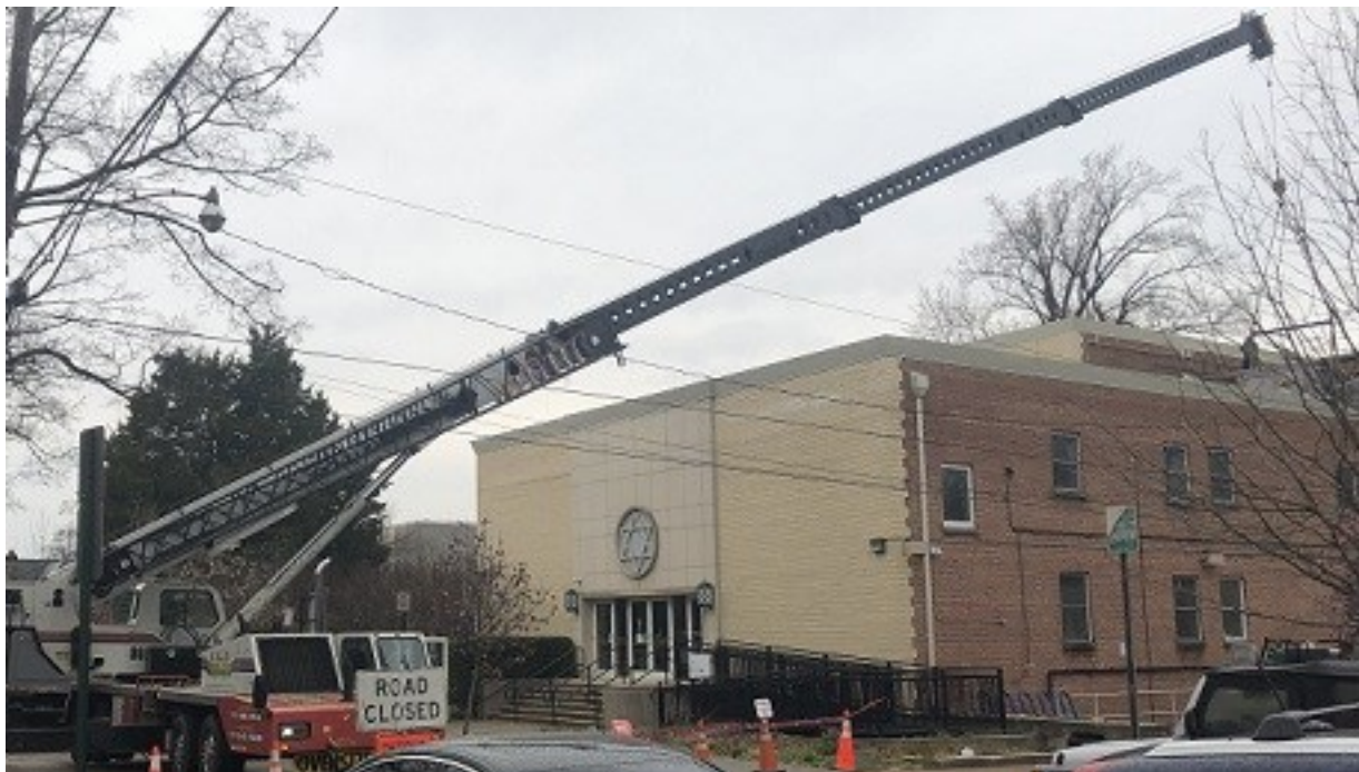
Crane preparing to lift our new air-handling equipment into the building via the roof. Photo by Sheri Blonder.
