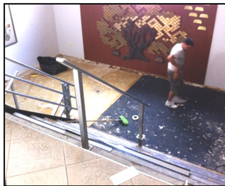
Carpet installer works on landing after stripping stair treads and old carpet
